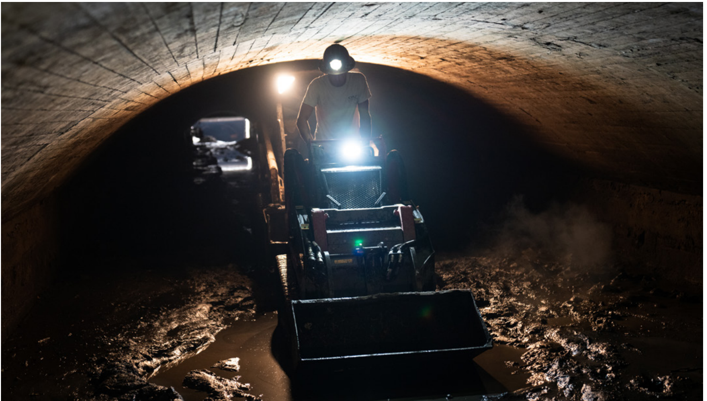
Figure 2. A worker uses a skid loader to remove sediment from the Old Bassett Creek Tunnel in Minneapolis.
