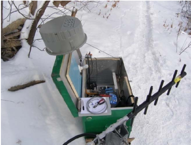
Figure 10. Monitoring Equipment Cabinet at a Mississippi River Stormwater Outfall
